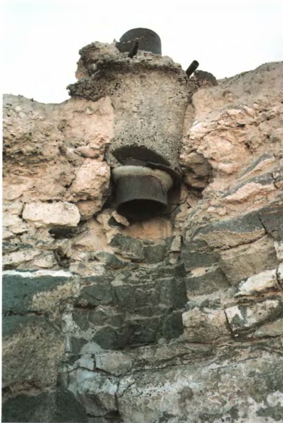
Road cut near Kimberly, Idaho reveals a cross section of an open-hole well construction frequently used in Idaho. Surface casing is cement grouted to the well borehole to a shallow depth. The remaining borehole is left uncased, allowing mixing of water from aquifers throughout the depth of the well. (Photograph by D.J. Parlman, U.S. Geological Survey.)
