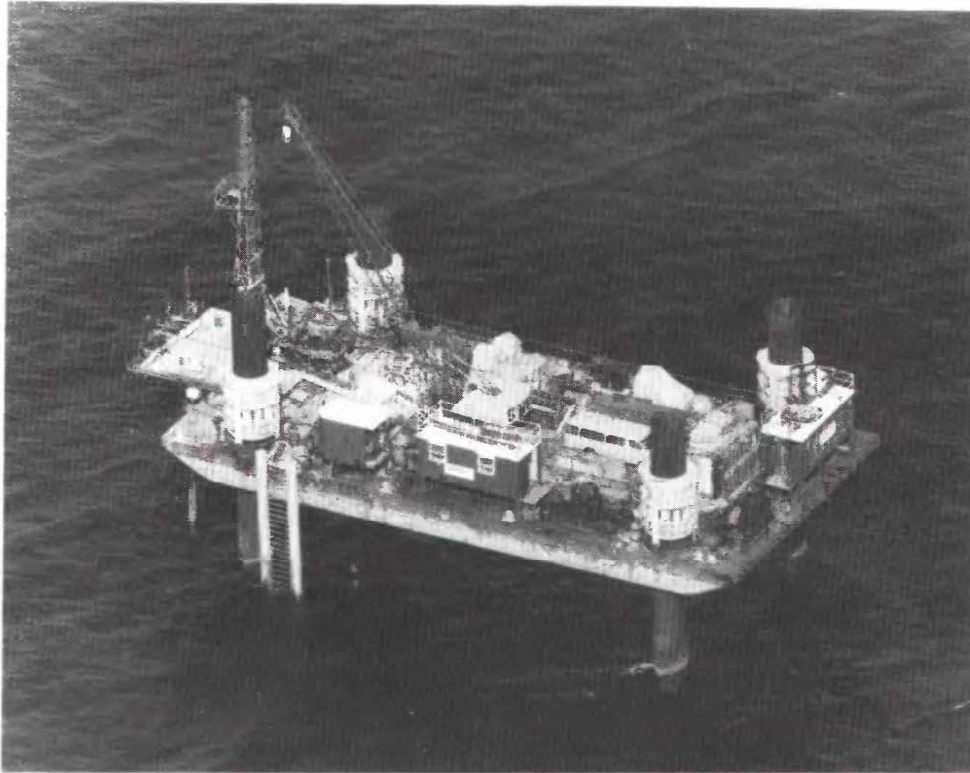
Water well drilling offshore of Atlantic City, New Jersey, summer 1985. The U.S. Geological Survey, in cooperation with the New Jersey Department of Environmental Protection, drilled two deep observation wells 1.9 and 5.3 miles offshore to evaluate the likelihood of saltwater intrusion toward onshore freshwater supplies. At these respective sites, the wells were drilled to depths of 933 and 1,025 feet below the sea floor. Dissolved solids increased seaward, but freshwater was found in both wells.
