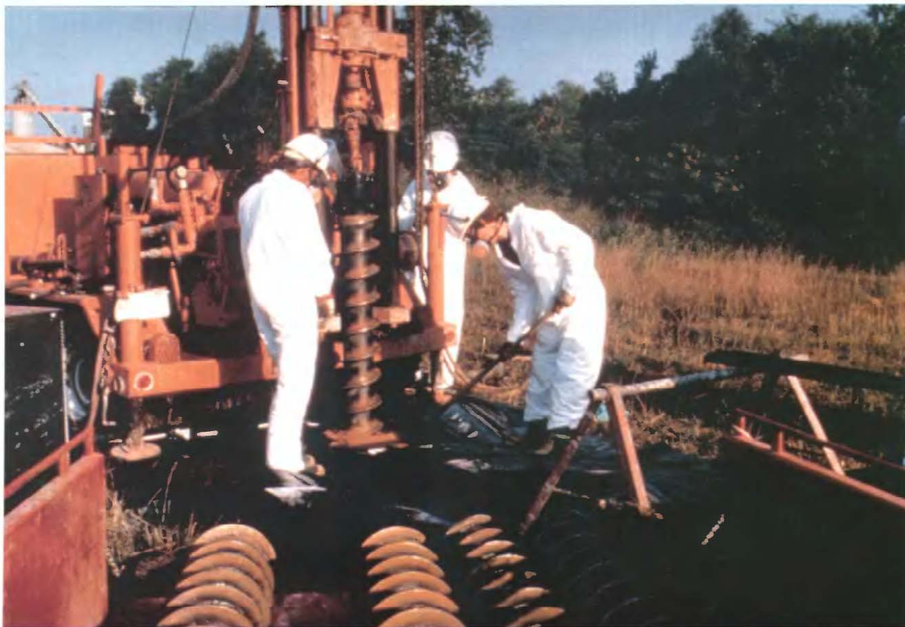
Drilling operations at a hazardous-waste site in west Tennessee. The U.S. Geological Survey in cooperation with the City of Memphis installed monitor wells at the Hollywood Dump in Memphis, Tennessee to evaluate the extent of ground-water contamination in the shallow unconfined alluvial aquifer beneath the site. All of the water being used for municipal and industrial supplies in Memphis is derived from deeper confined aquifers. (Photograph by David D. Graham, U.S. Geological Survey.)
