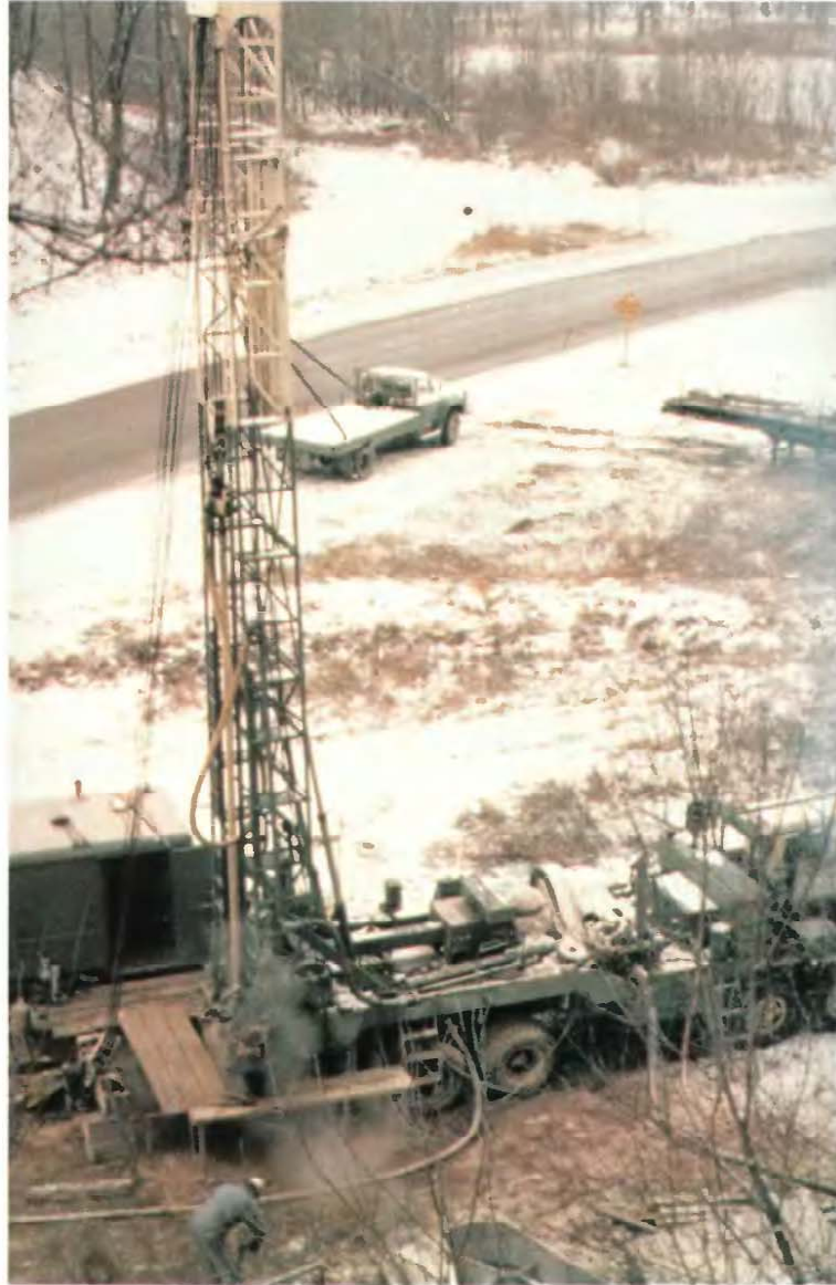
Drilling a deep test well in southwestern Wisconsin. This well was used to measure hydraulic head and water quality differences between individual units of the sandstone aquifer. (Photograph by James T. Krohelski, U.S. Geological Survey.)
